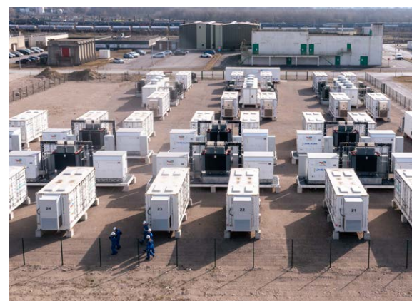
The battery energy storage site in Dunkirk © Redfox - Redfox - TotalEnergies
